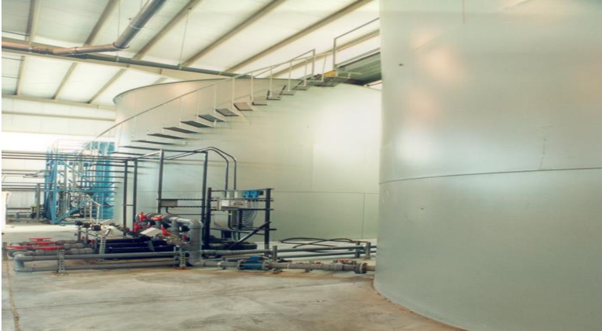
PDS fermentation and storage at 26 th Ward WPCP in New York City, 2002
